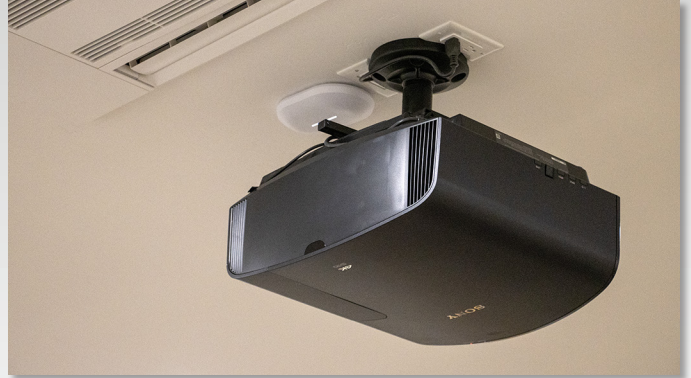
AP6-Pro Installed in Home Theater
