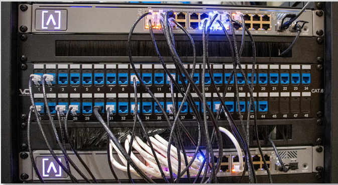
Network Rack with 2 S24POE Switches
