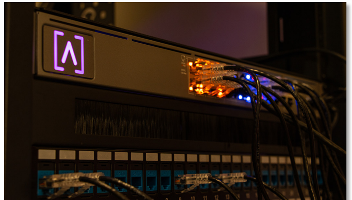
S24-POE Switch Installed
