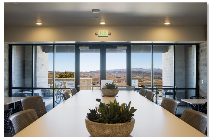
AP6-Pro Installed in Community Room
