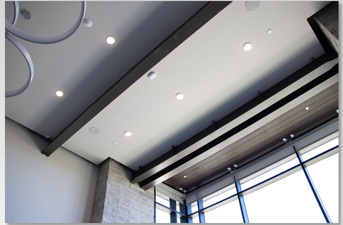
AP6-Pro Installed in Main Lobby
