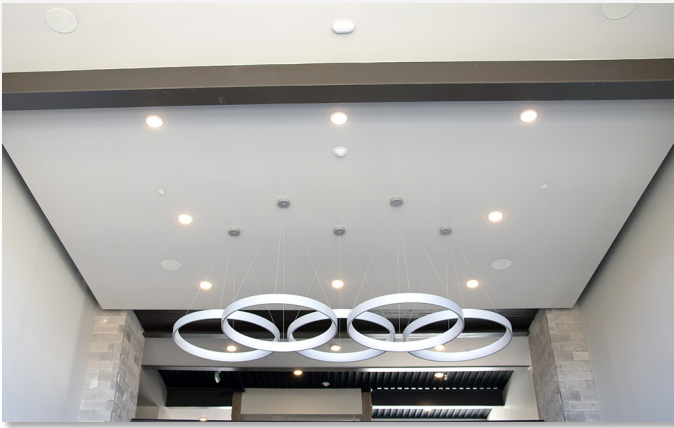
AP6-Pro Installed in Main Lobby
