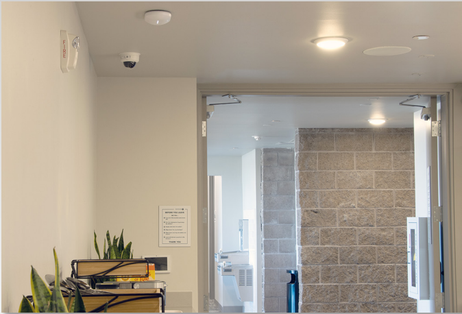
AP6-Pro Installed in Kitchen
