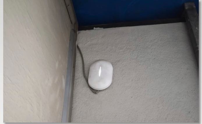
AP6 Deployed in the Warehouse
