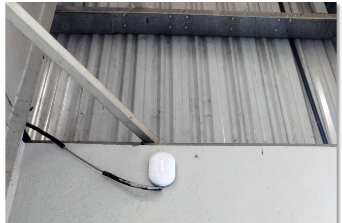
AP6 Mounted in the Warehouse
