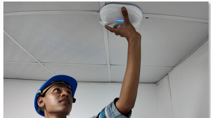
Replacing a UniFi AP with an AP6-Pro
