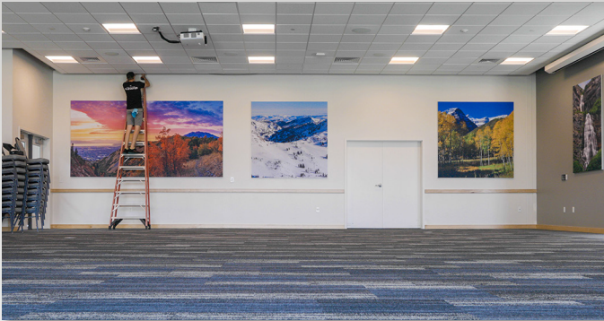
Installing an AP6-Pro
