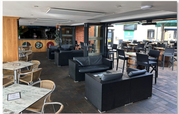
AP6-Pro Installed in the Viking Bakehouse/Tiki Bar
