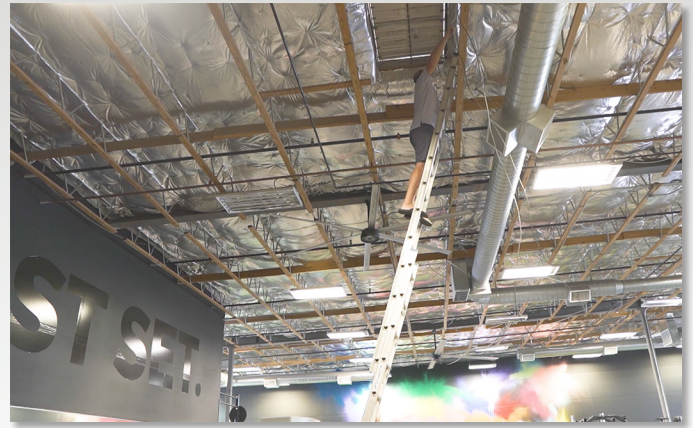
AP6-Pro Installation Above the Fitness Culture Gym
