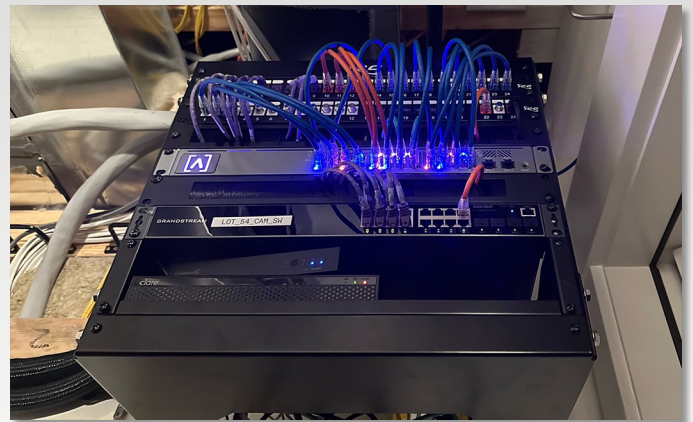
Alta Labs S24-POE Switch Installed in Closet
