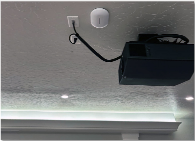
AP6-Pro Installed Near Projector in Home's Theater
