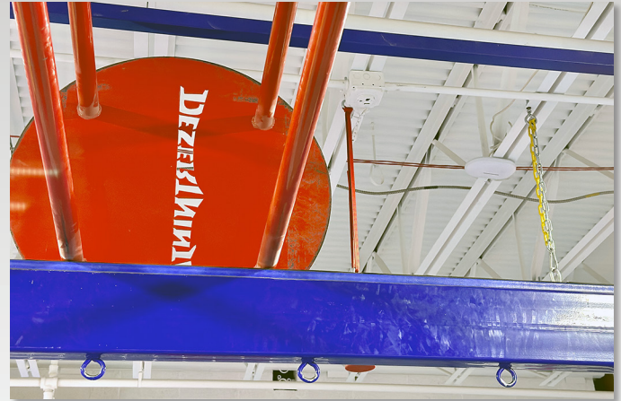
AP6-Pro Installed Above The Gym at the Be More Complex
