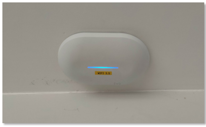
Closeup of AP6 Installed
